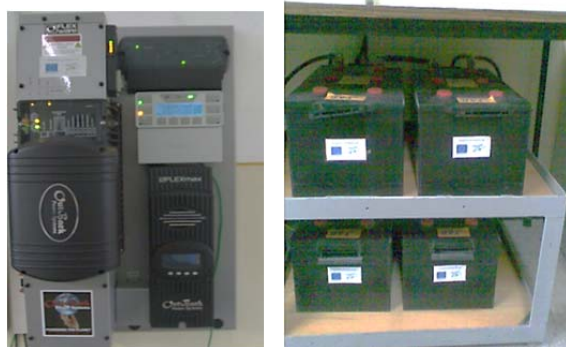
Fig. 3. The inverter-battery ensembles.
