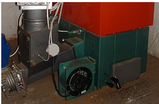
Fig. 3. View of an air distribution box
